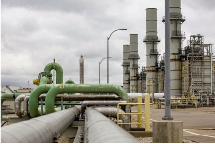
Corp.'s Midlothian Power Plant. State leaders announced Monday that Texas will double a fund aimed at spurring the construction of more gas-fired power plants as power demand is projected to increase sharply. Photo Credit: Shelby Tauber for The Texas Tribune
